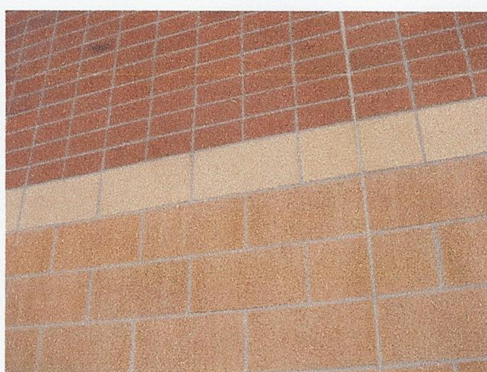
16" thru wall brick laid in standard half bond with 50/50 slot to give stack bond appearance (Living Hope Church, Frankfort, IL)
