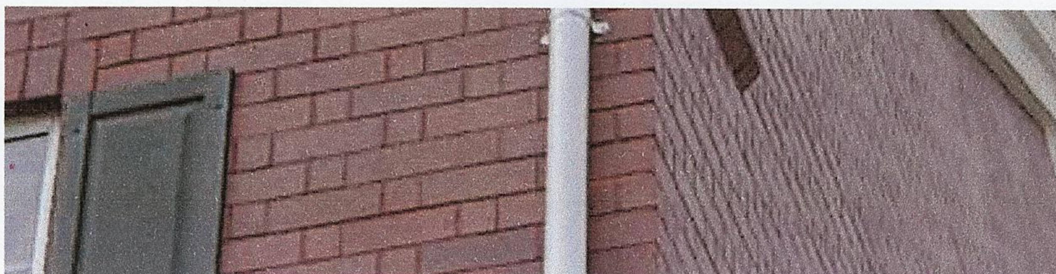
This client could not afford to have their mason lay a Flemish bond pattern. Once they switched to a slotted brick (2 1/4" x 12"), they saved enough money to upgrade some other areas of their project!
