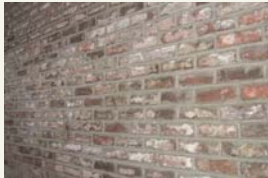
Reclaimed street pavers used as an external material. L.L. Bean- Barrington IL.
