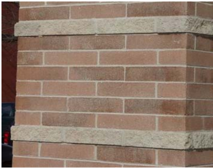
A pillar made of brick. The sun's UV rays and other weathering have impacted its color.
