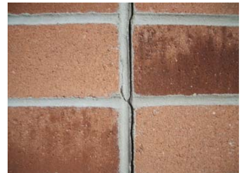
Fading color and shrinking: 2 big reasons to reconsider using CMU
